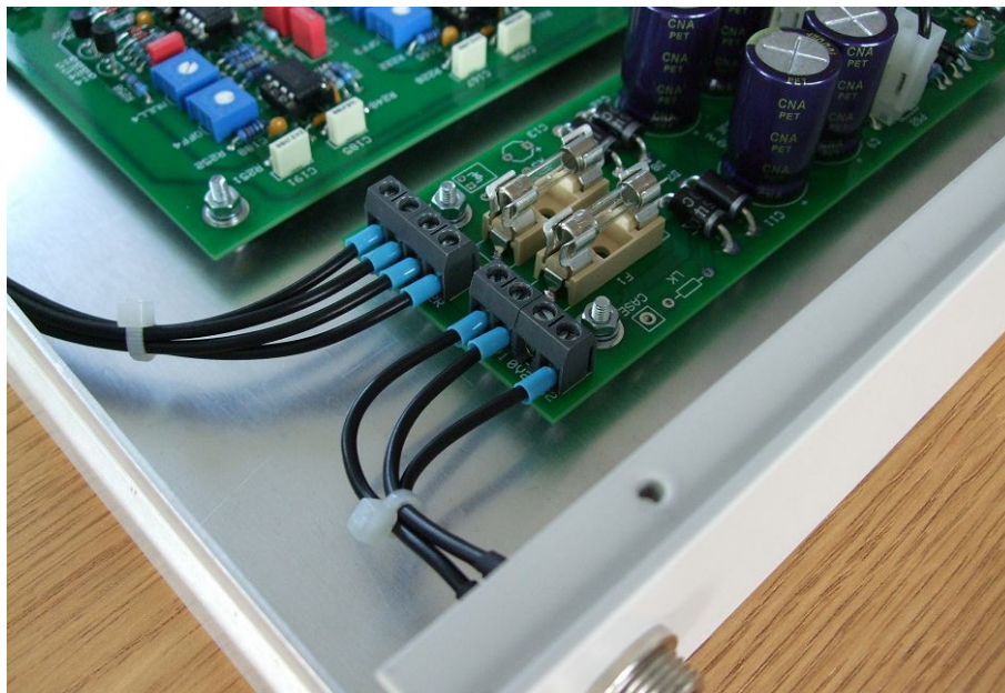
All power wiring uses 24/0.2 insulated wire. I have also boot lace ferrules on the wire ends that go into the terminal blocks for neatness.
